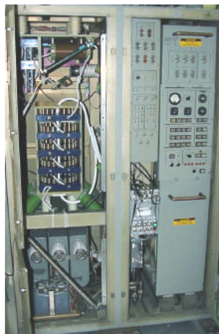
Fig. 6. Solid-state cathode-pulsed, prototype modulator in SPS-49 transmitter.
